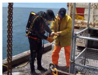
Divers preparing to remove debris from under the wharf prior to dredging
