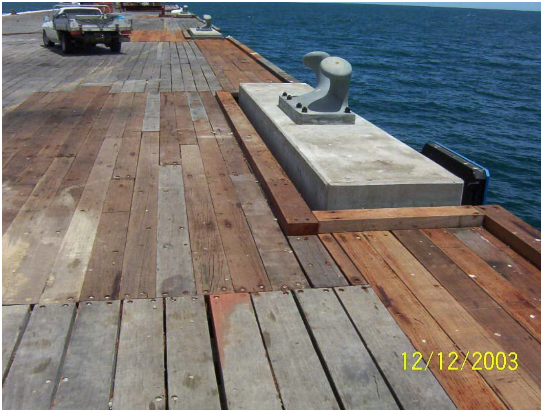
Wallaroo- all ten new berthing and mooring dolphins completed- ready for shipping
